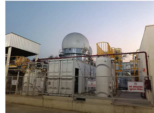
Biogas plant installed at the Manesar Plant
